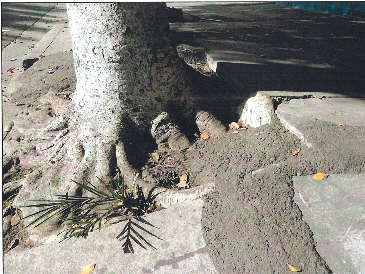
Extensive surface roots from ficus tree no. OS-2 that are causing destructive damage to surrounding sidewalk and city hardscape.
