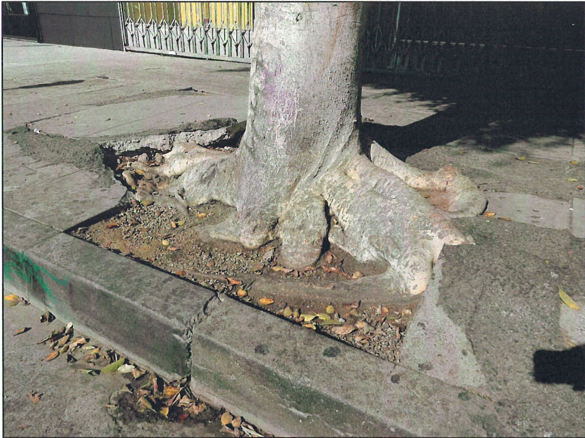
Extensive surface roots from ficus tree no. OS-4 that are causing destructive damage to surrounding sidewalk and city hardscape.
