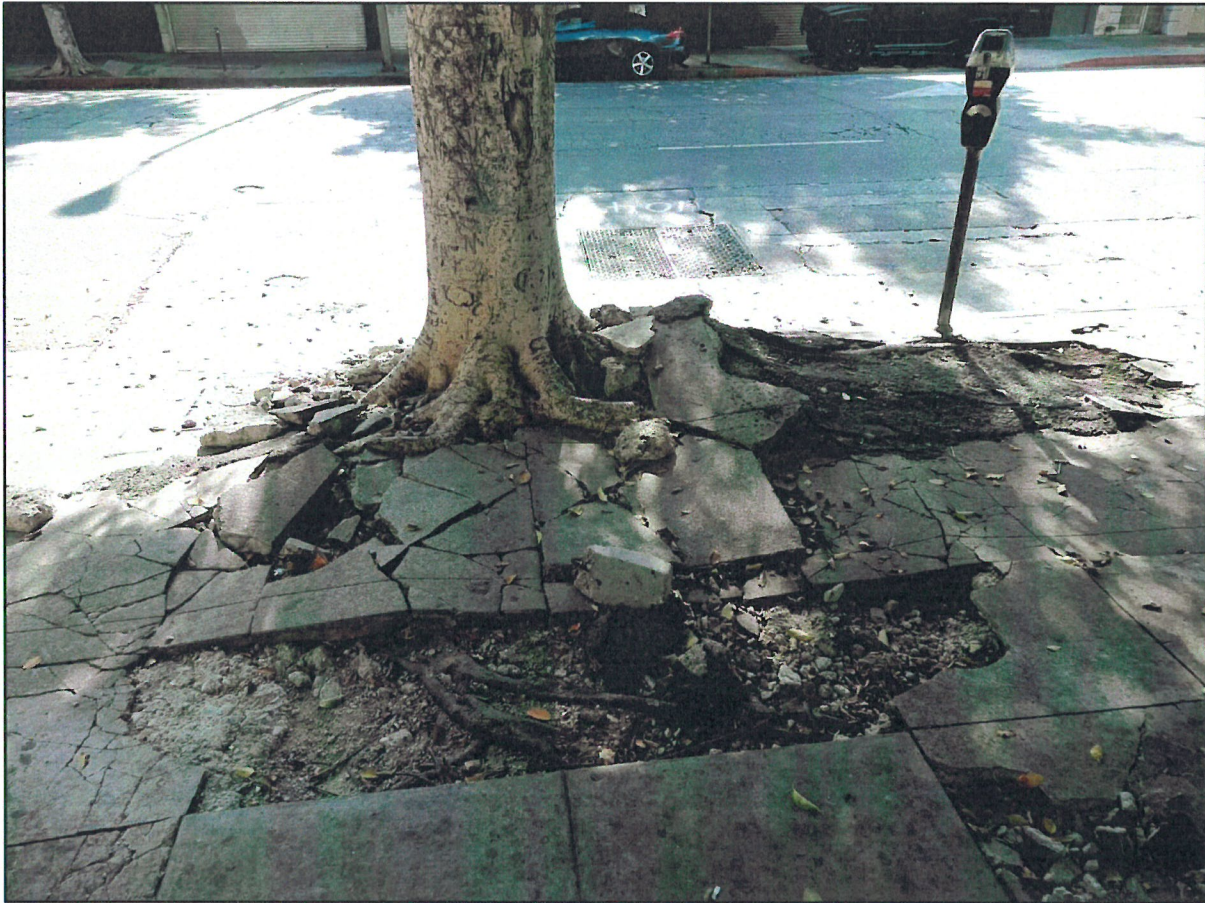
Extensive surface roots from ficus tree no. OS-3 that are causing destructive damage to surrounding sidewalk and city hardscape.
